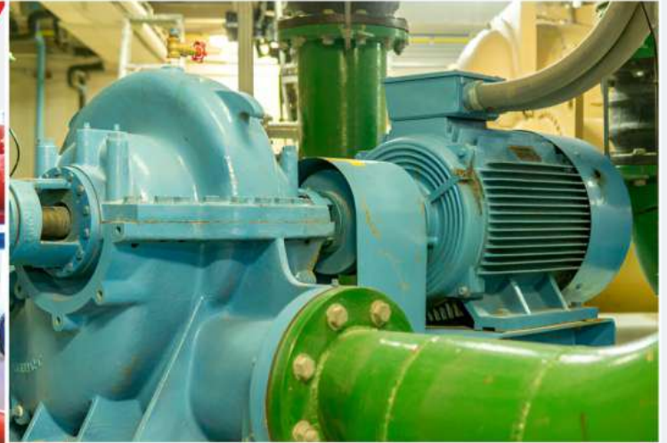
Horizontal Shaft Laser Alignment
